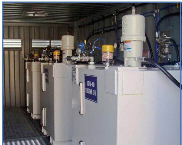
Figure 4 – Inside the Three Tank Container
