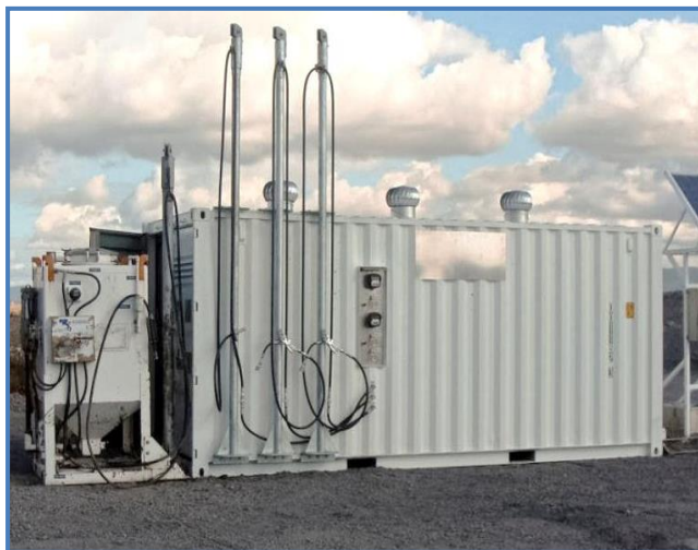
Figure 1 – IRS Remote Storage, AS1940 Compliant System
