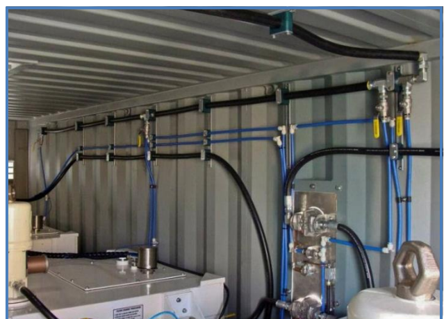
Figure 5 – Hose and Gauges Set Up
