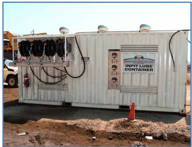
Figure 2 – IRS 20 Foot Remote storage with Hose Reels
